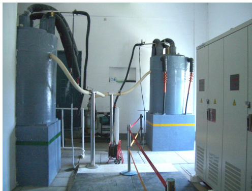
Figure 3. The 10.5 kV/1.5kA SFCL installed at a substation.
